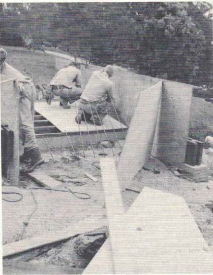
Mr. Church and fellow carpenters build the wood forms for a graceful concrete bridge over the stream.
