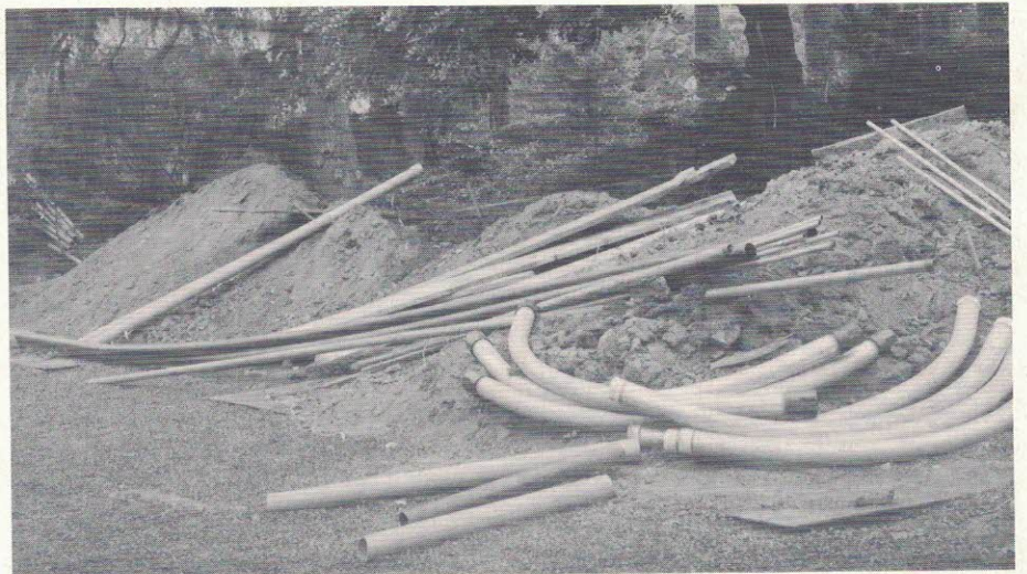
Along with the water pipes went these electrical conduits—now unifying the upper-campus electrical system.
