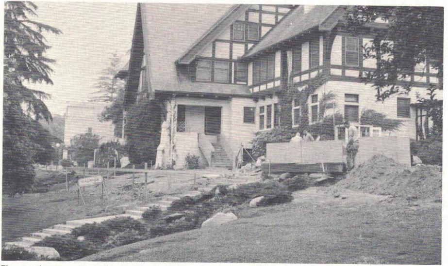
The northeast corner of Mayfair is undergoing a face-lifting. Between the caution sign and the north corner will be a large patio.
