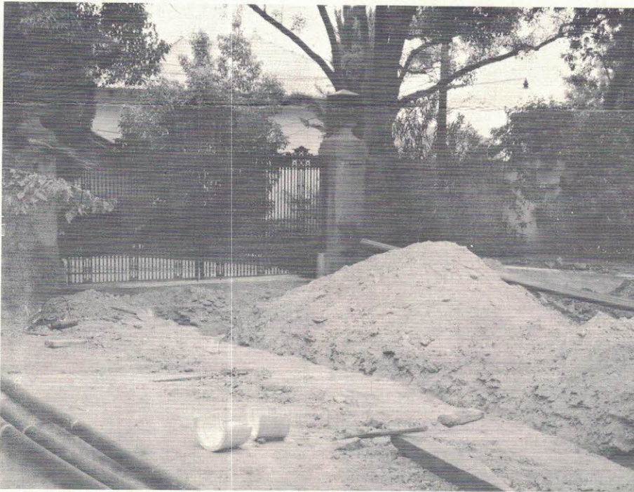
As far as the parking lot in front of Ambassador Hall, the ground is opened for the campus-long water main.
